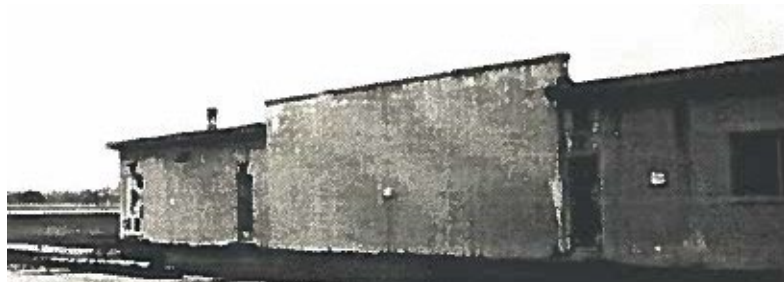
Building 98 from the road, with the large wall available for a sign. (Don Saunders photo)
